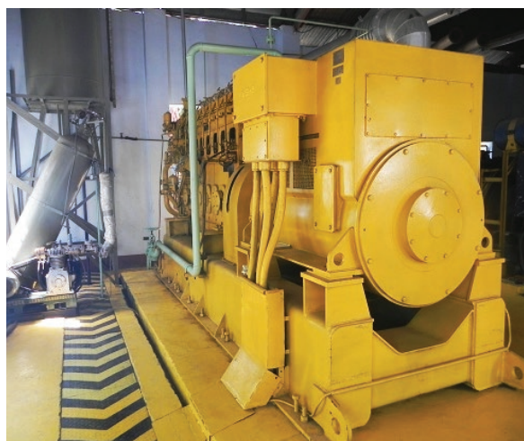
NPC-SPUG Diesel Power Plant Unit No. 5 in Ticao, Masbate (Photo credit: NPC)
