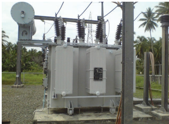
Pad-mounted transformer in Southern Palawan substation of NPC-SPUG
